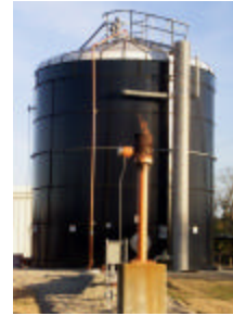
Fixed film digester
